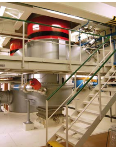
Spalovňa Incineration facility
