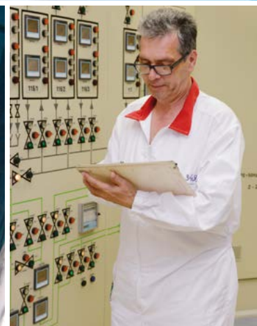
In the control room of the Interim Spent Fuel Storage
